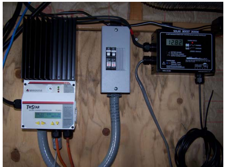
Here is a picture of my solar control panel. The 45 amp charger is on the left. The 25 amp charger for the 24 volt system is on the right. The circuit breaker box in between has DC breakers to separate the batteries and solar panels from the chargers. Small wires exiting each charger are for temperature compensation of the batteries. A temperature sensor gets clamped on a battery terminal and lets the charger know how warm or cold the battery is. This allows proper charging at all temperatures, winter and summer. Note the plastic strain reliefs for the DC wiring.
